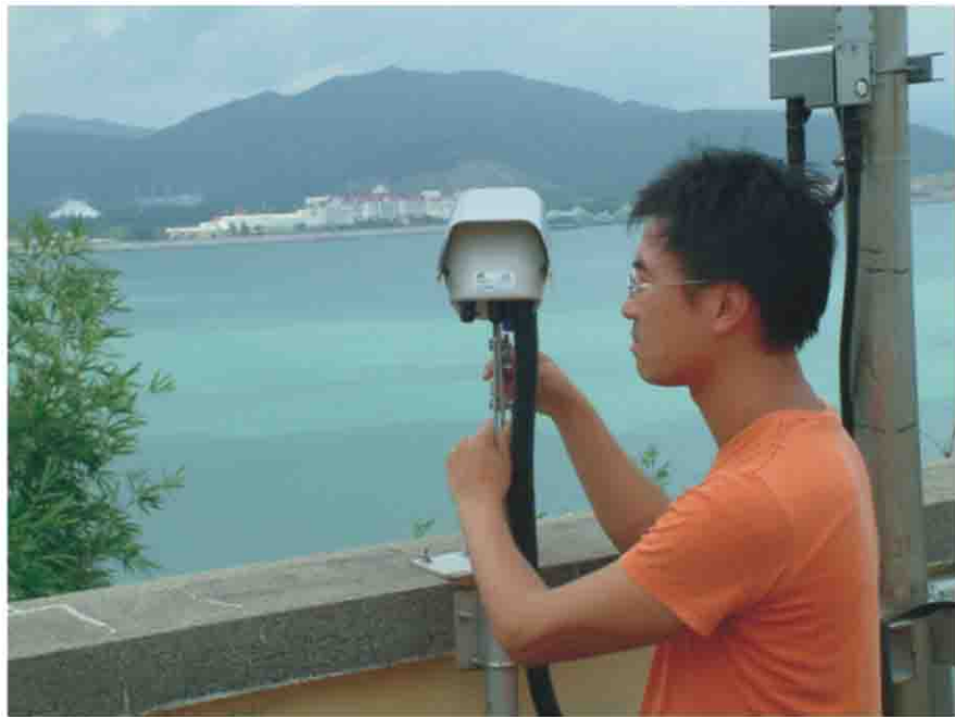
Mr IP Chi-wing, Radar Specialist Mechanic, installing an automatic camera at Peng Chau
