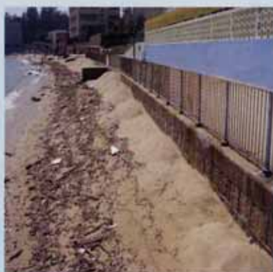
The beach at Cheung Chau was eroded by the storm surge associated with Typhoon Hagupit in 2008.
