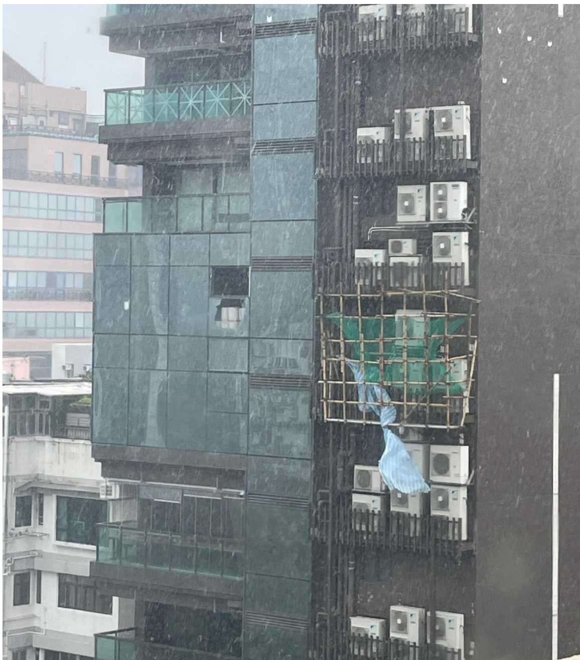
圖 2.2.17 樺加沙襲港期間，尖沙咀有大廈的玻璃幕牆受損。(鳴謝：呂旭昇) Figure 2.2.17 During the passage of Ragasa, the glass curtain wall of a building in Tsim Sha Tsui was damaged. (Courtesy of Lui Yuk Sing)
