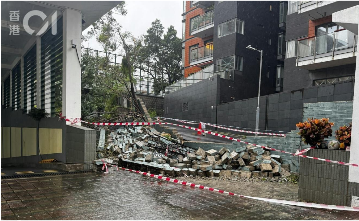
圖 2.2.15 樺加沙襲港期間，九龍塘有小學的圍牆倒塌。(鳴謝：香港 01 / 林振華攝) Figure 2.2.15 During the passage of Ragasa, the wall of a primary school in Kowloon Tong collapsed. (Courtesy of HK01 / Photo by 林振華)
