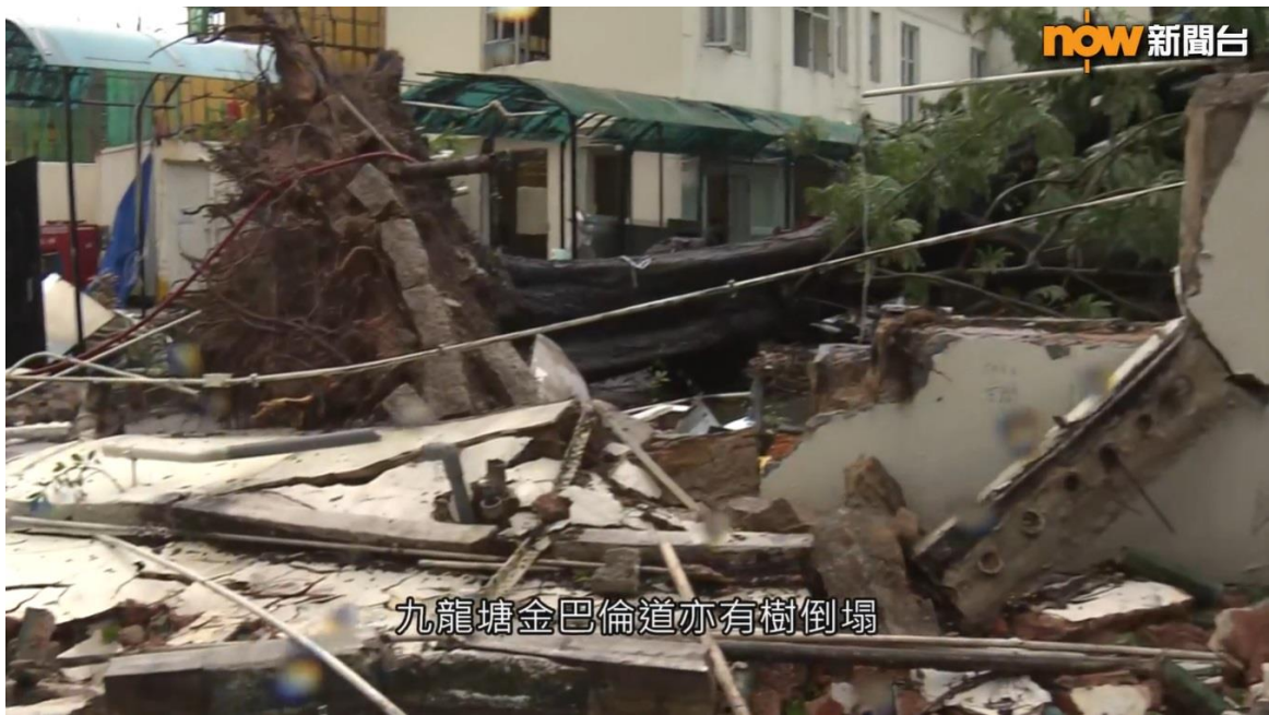
圖 2.2.16 樺加沙襲港期間，九龍塘有獨立屋的外牆被塌樹壓毀。(鳴謝：Now 新聞) Figure 2.2.16 During the passage of Ragasa, the wall of a detached house in Kowloon Tong was damaged by a fallen tree. (Courtesy of Now News)
