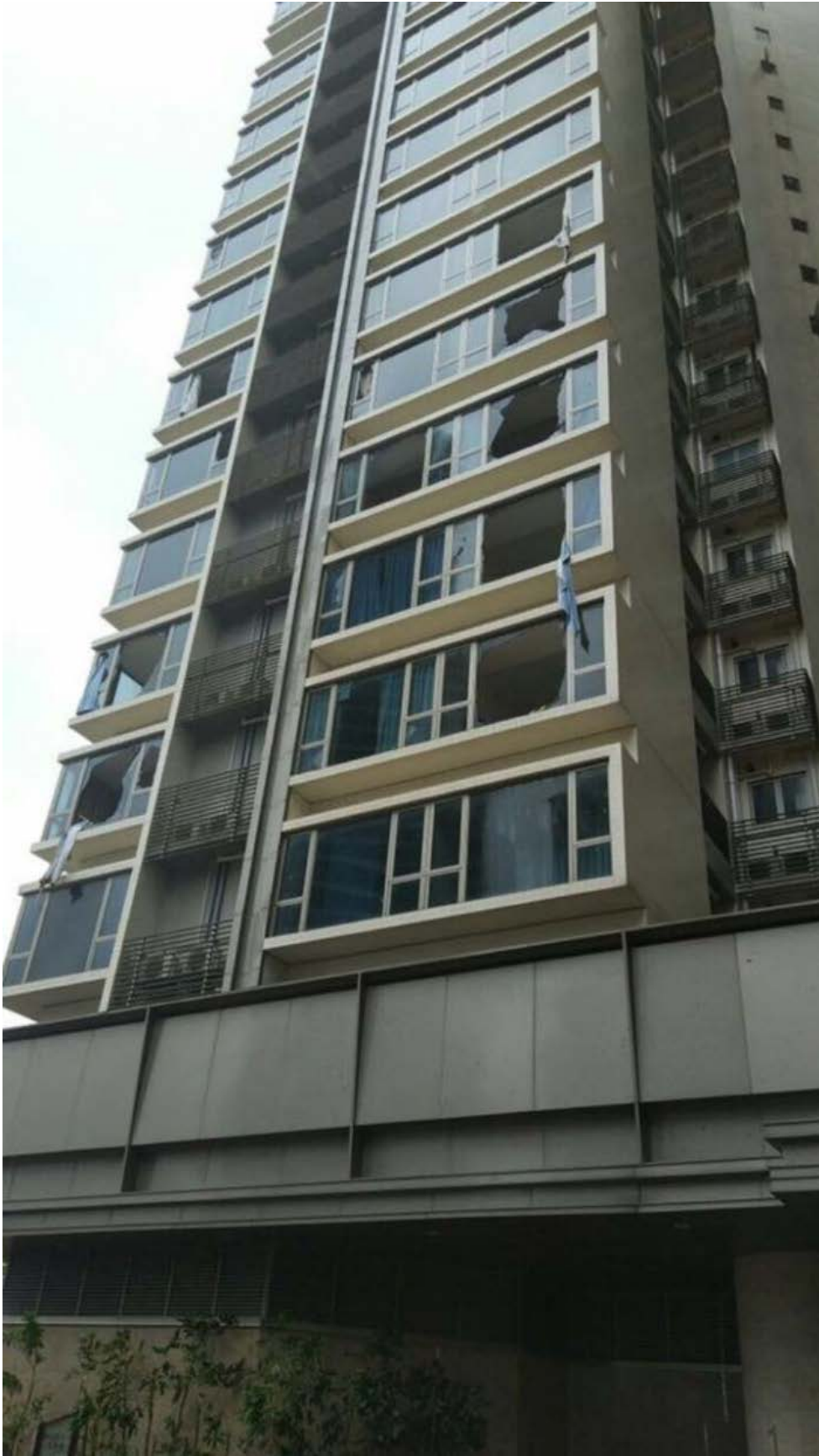
圖 3.3.21 澳門有住宅大廈的窗戶玻璃爆裂。(圖片鳴謝: 方志剛) Figure 3.3.21 Window panes of residential buildings in Macao were broken. (Photo courtesy of Clarence Fong)
